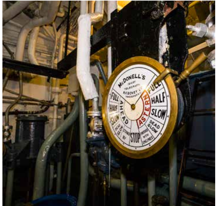
Adjacent to the throttle handwheel is the engine room telegraph, which relayed orders from the wheelhouse.
